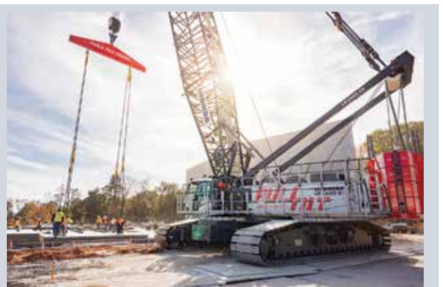
Full Tilt Crane Services added a 400 tonne Liebherr LR 1400 SX to its fleet to lift larger and heavier panels
