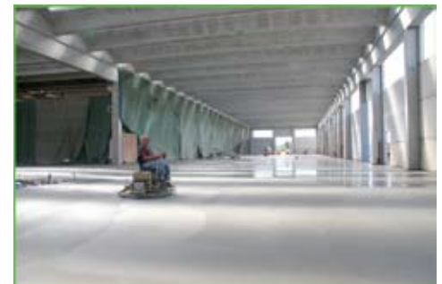
A factory extension nearing completion, which will double the size of the Tre Emme company (above).
