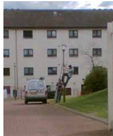
These tradesmen have some ladders but are still struggling to reach the lamp. Clearly some common sense training is required.
