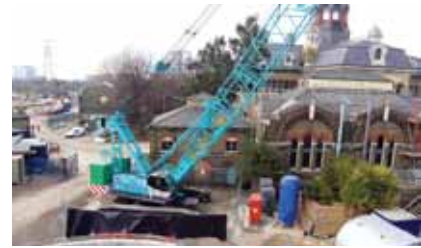
Q-Plant's new 135 tonne Kobelco CKE1350 at the Abbey Mills pumping station in East London.
