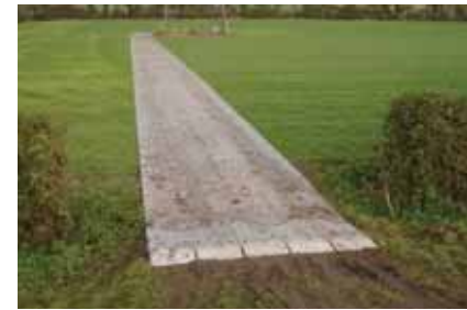
Aluminium road ways from companies such as TPA, Eve and Timbermat are well suited for wheeled cranes and lifts to gain access over soft ground.
