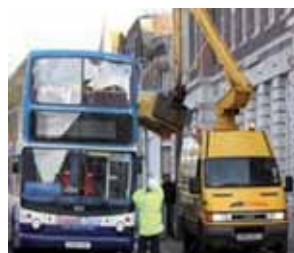
Clearly the set up for this job was well below par, and could so easily have resulted in a fatality.
