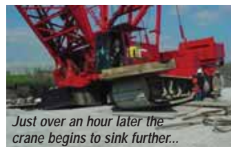
Aggregate platforms need to be carefully calculated and built or they can easily give way
