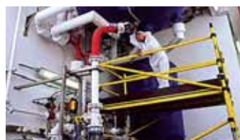
New applications for towers are still being found.
