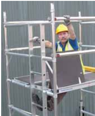
The guardrails for the next level are installed through the trap door before climbing onto the platform.
