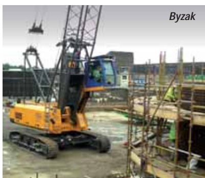
The Sennebogen 660 works on cantilevered falsework to carry out a wide variety of tasks
