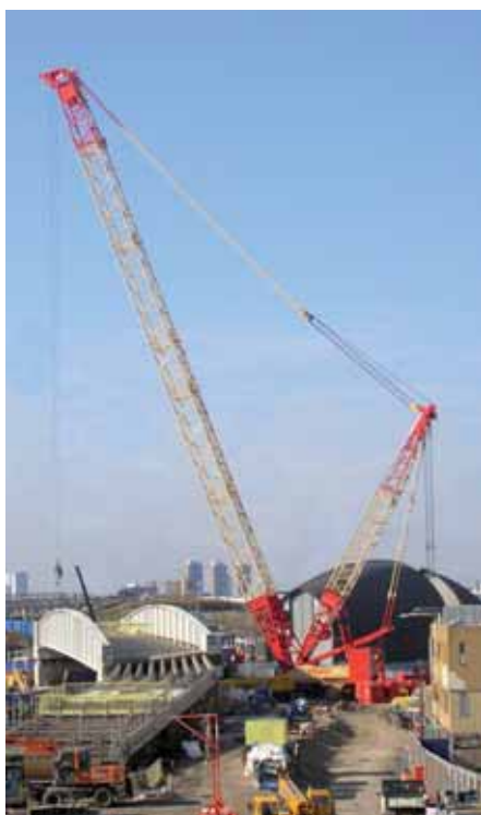
The Weldex 550 tonne capacity Kobelco SL6000 with 72 metre main boom in Super Heavy Lift configuration, installing the pre-cast abutments and the two main prefabricated steel span beams weighing up to 110 tonnes each.
