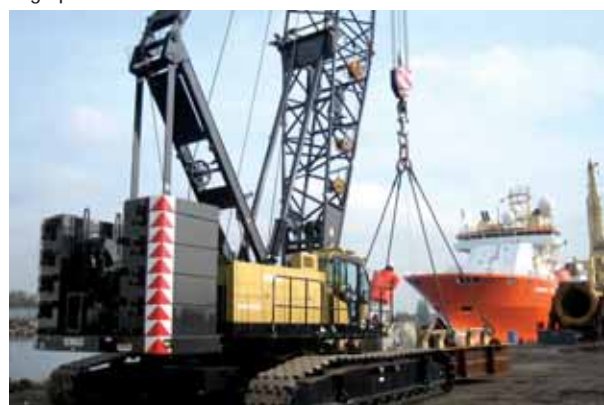
The Kobelco CKE1350 being prepared and tested at the Saipem dock-side yard in Schiedam, Netherlands, before being transferred by barge to the Saipem 7000.
