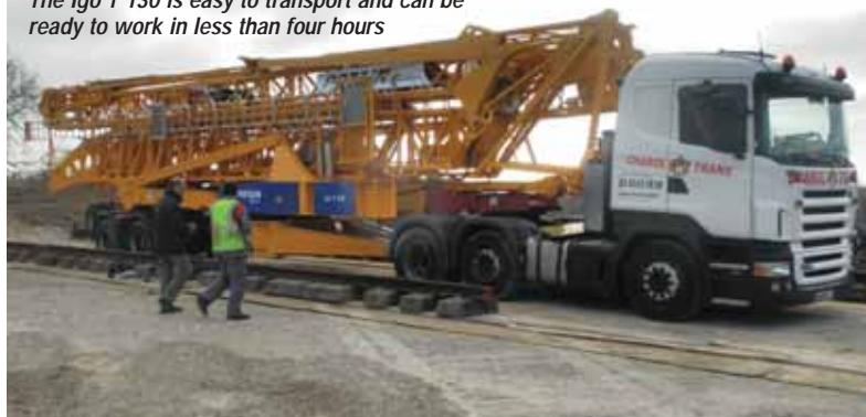
Five Linden Comansa 21 LC290 18 tonne cranes are being used to construct the bridge pillars for the 37km long Necaxa to Avila Camacho section of the Mexico-Tuxpan highway
