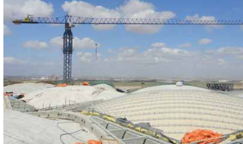
Three Linden Comansa 21 LC 400 flat top cranes are carrying out the work at Amman airport in Jordan
