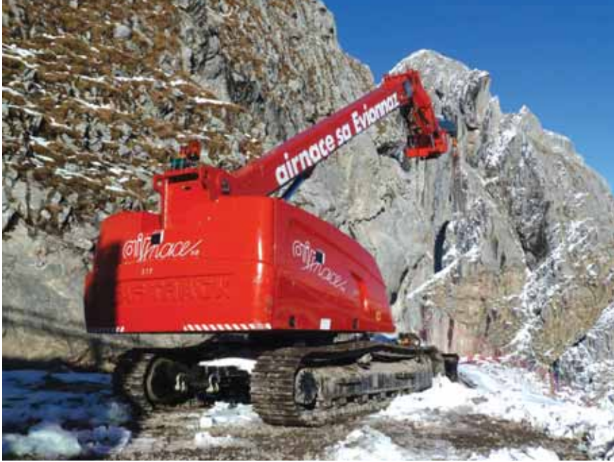
The Giraf Track travelled 10km up exceptionally steep mountain tracks to reach the job site.
