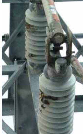
An insulator damaged from flash past
