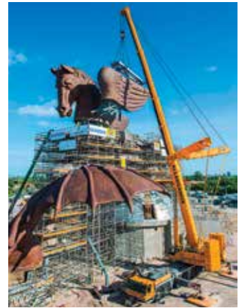
A seven axle, 400 tonne Liebherr LTM 1400-7.1 AT crane operated by Allegiance Crane of Pompano Beach was used.
