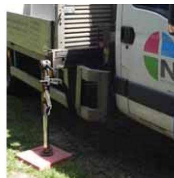
The mat on the unloading side on the dry lawn. At the rear a mat was used on interlocking blocks - not necessary but still good practice.
