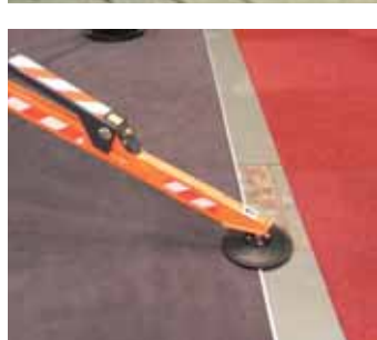
While the indoor floors at APEX are solid, there are voids, many of which are hidden by carpet.
