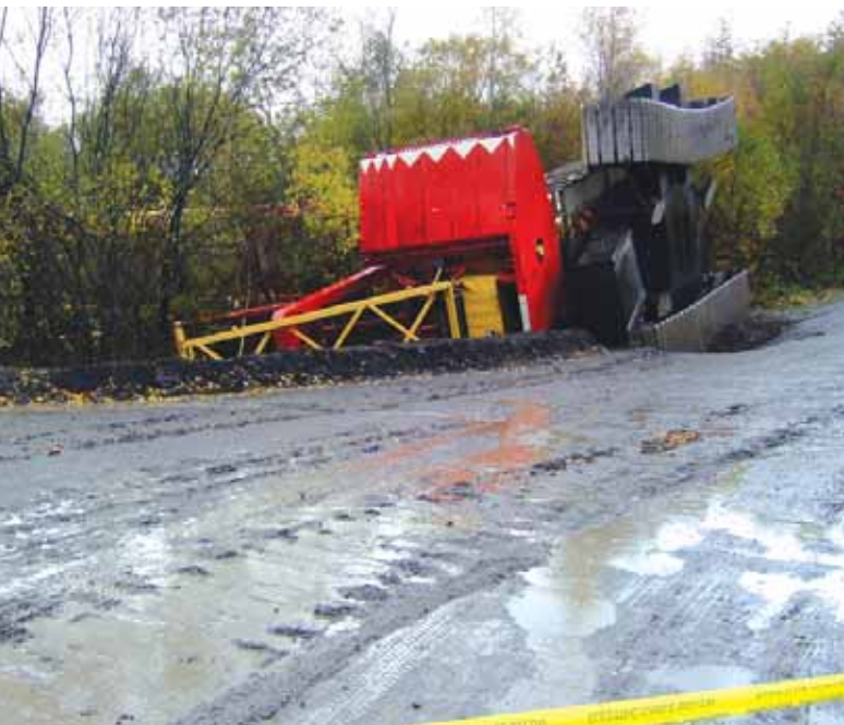
This crane went over when the road collapsed while travelling fully rigged.
