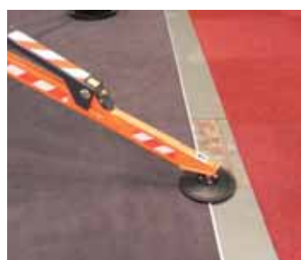
While the indoor floors at APEX are solid, there are voids, many of which are hidden by carpet.
