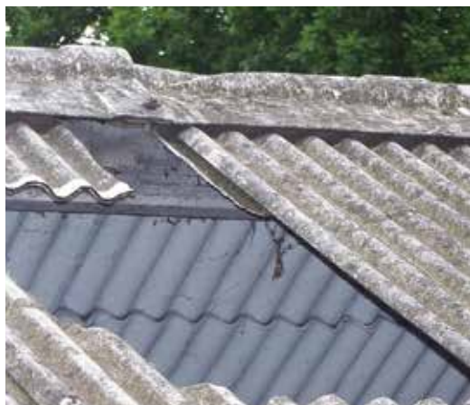
Andrew Ward fell more than eight metres to his death through a fragile cement roof
