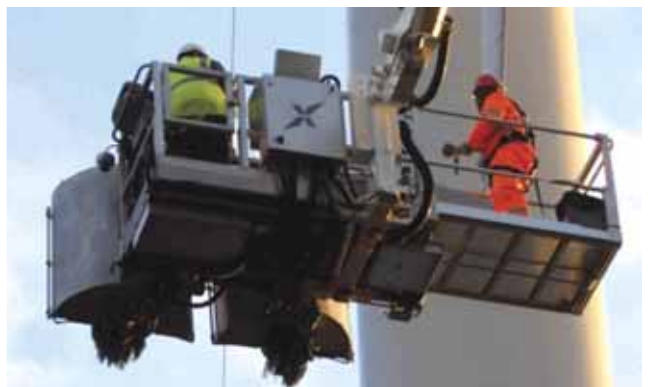
If a blemish is spotted on the blade specialist cameras carried on the platform extension can be deployed
