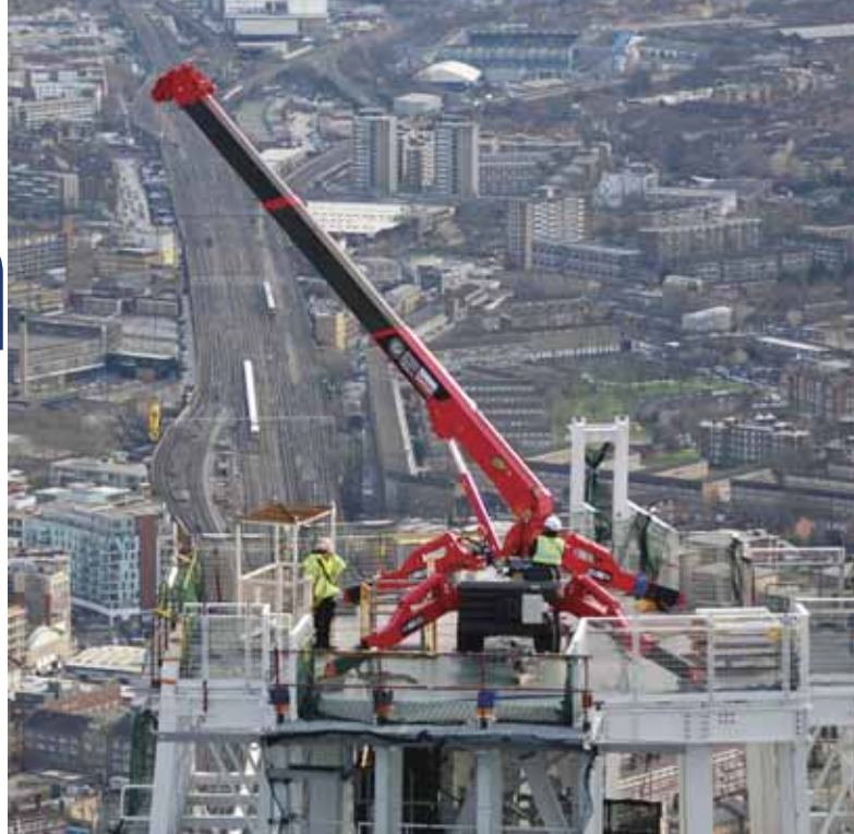
Up goes the base crane - all the way to the 87th floor
