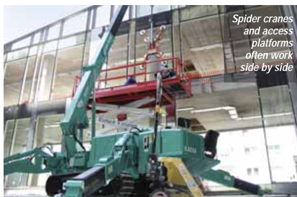
Being able to access canal locks along the tow path is a major advantage for the spider crane
