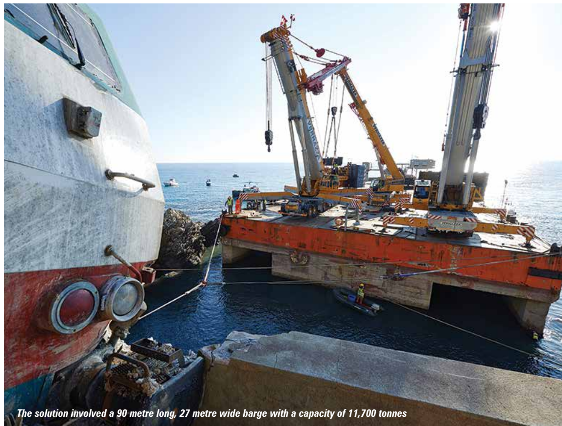
The derailed train stuck between the cliffs and sea
