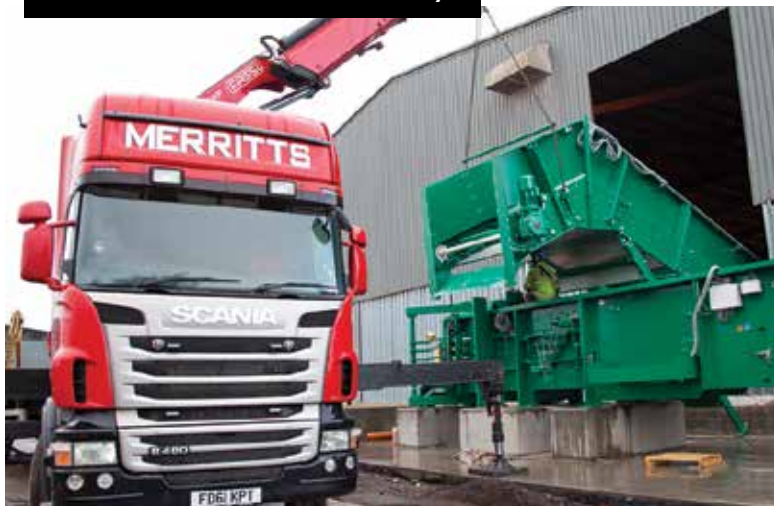
The Fassi F660XP and Versa-Lift fork lift were used to install the horizontal baler and incline conveyor
