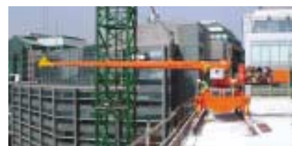
Mini cranes are ideal for roof applications, here a custom built rail mounted Imai is used to place windows below.
