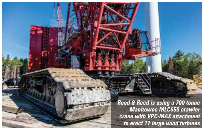
The MLC650 is rigged with 128 metres of boom and a 7.6 metre offset upper boom point, providing an overall tip height of 137 metres
