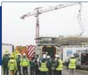
A tower crane collapsed killing two employees
