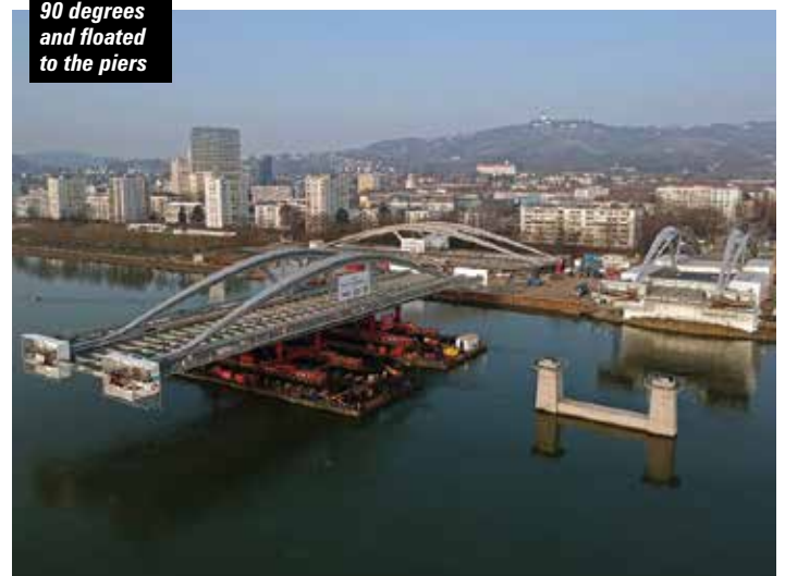
The bridge was moved by the four SPMT sections on to the two double barges
