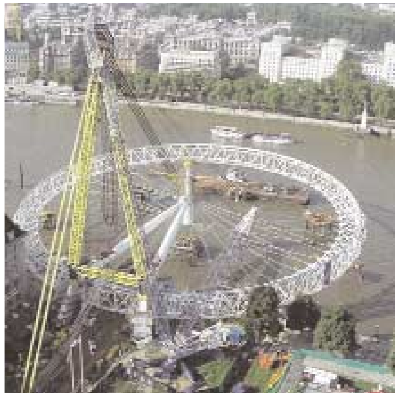
Jobs such as the lifting of the London Eye and the salvaging of the sunken Russian submarine, the Kursk, have helped give Hydrosplex a reputation as a pioneer of advanced alternative lifting systems.
