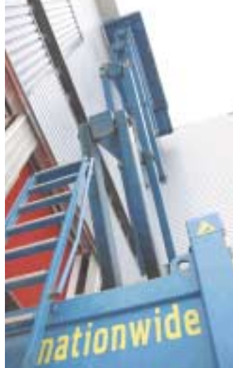
Nationwide Access recently supplied this 28-metre, 16-tonne diesel powered Liftflux LL26X to Donkin Roofing for cladding work on a 25-metre high steel framed bay pallet storage warehouse at Tilbury Docks.
