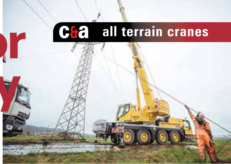
Crane Maier used its new Liebherr LTM 1070-4.2 to replace aging high voltage pylons for Deutsche Bahn
