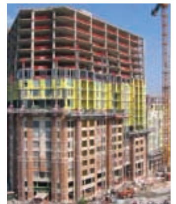
Scaffolding for a 10- to 12-storey block on four sides can take up to four to five weeks to erect and up to four weeks to dismantle. To cover the same building with MCWPs would take about a week.
