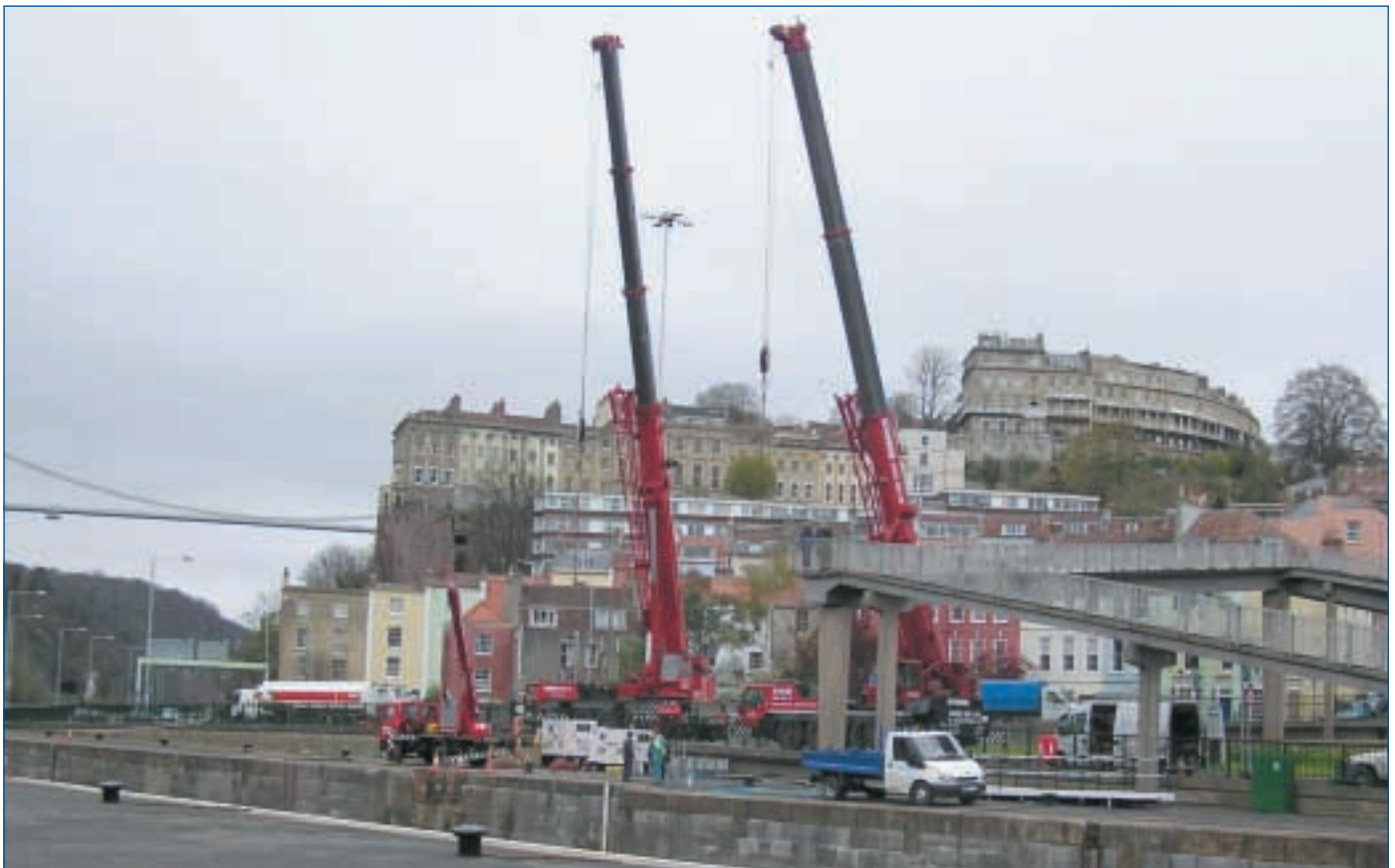
The Clifton Suspension Bridge in Bristol formed the backdrop to a lift performed by Sparrow Crane Hire recently, which was called in by Bristol City Docks to assist in the re-fitting of 90 tonne lock gates at the Cumberland Basin in the Avon Gorge. For the main part of the lift, Sparrow brought in a 100 tonne capacity Grove GMK 5100 and an 80 tonne Liebherr LTM 1080/1, (pictured), while supporting roles were provided by two Demag AC 40/1s and a Tadano TL 75.
