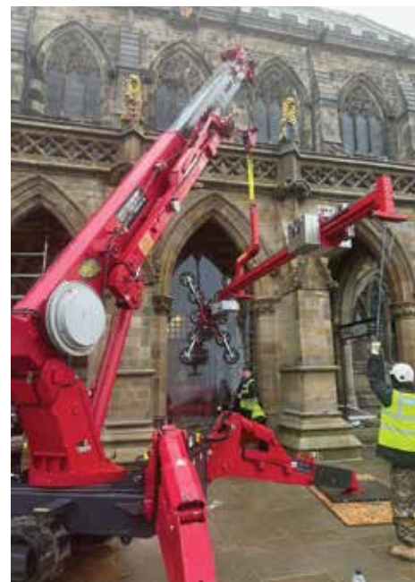
The Grade One listed Rochdale Town Hall installation required a Unic URW-706 spider crane with Libro 2500B overhang beam and GL-UMC1200 glass manipulating head
