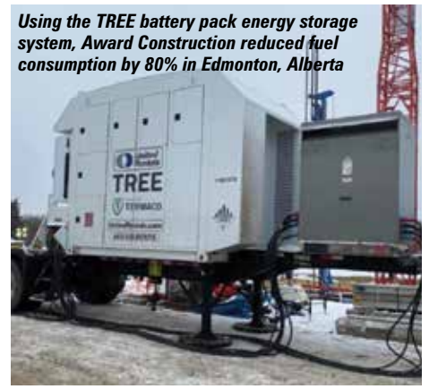
Radius delivers one of the AMPD Enerainer energy storage units
