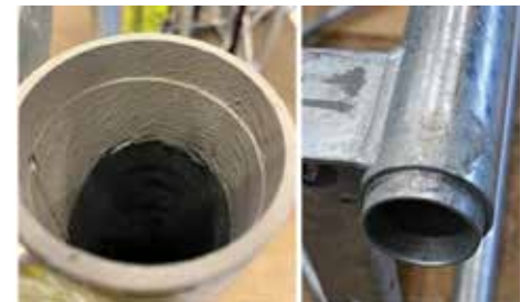
With critical bolts missing, the mast sections were only held in place by the friction between the short spigots and the sockets of the section below
