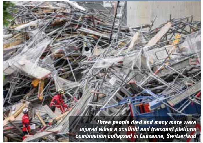
Five people died in Stockholm when a hoist car crashed to the ground from a height of around 20 metres
