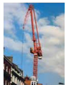
A Kroll 103V 'pipe crane' on a Skanska job in New Bond Street London
