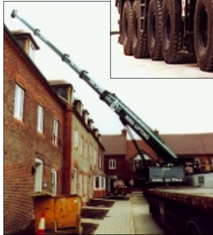
One of the first jobs for the new GMK6220-L was the placement of a 20 tonne footbridge at a new housing development near Salisbury
